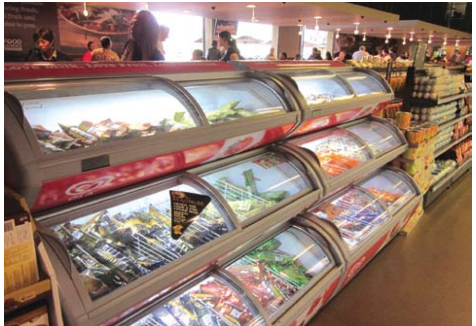
Traditionally, self-contained or plug-in cabinets were limited to smaller displays, such as ice cream at the check out. However, plug-ins are now a real option for regular cabinets in the rest of the store. Ultimately the decision is based on cost, capacity and efficiency.
