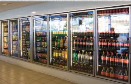
COLD / FREEZER ROOMS
