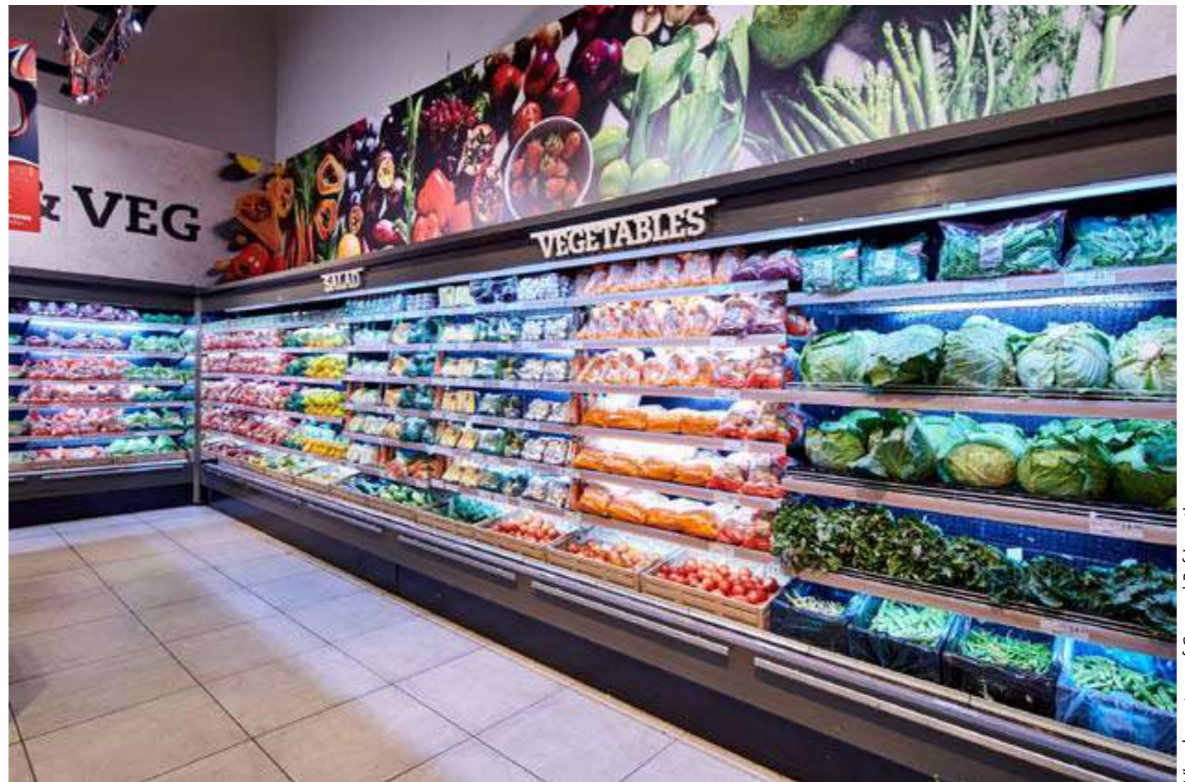
Visual courtesy of Concord Refrigeration
