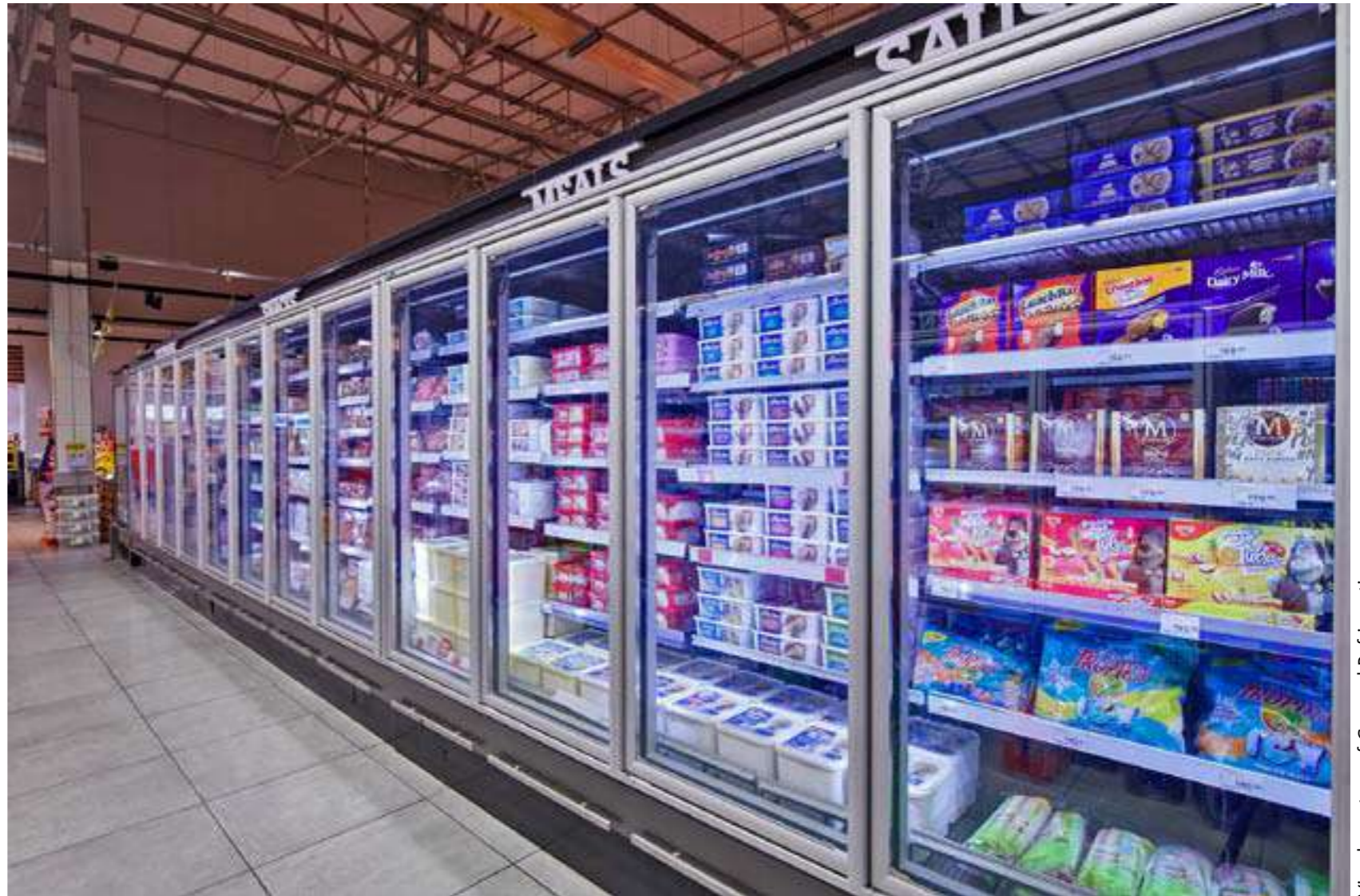
Visual courtesy of Concord Refrigeration
